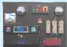
FAB (TPP) CONTROL PANEL
