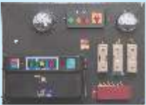
BSA (TPP) CONTROL PANEL
