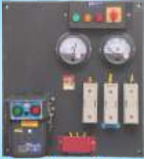
BOI (TPP) CONTROL PANEL
